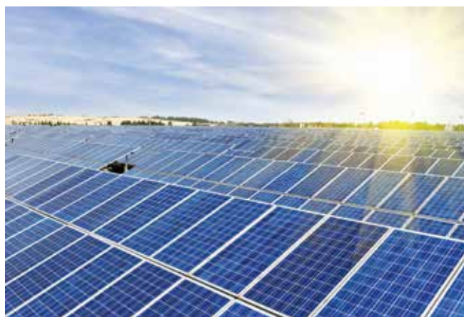
| Solar panels collect solar energy.
